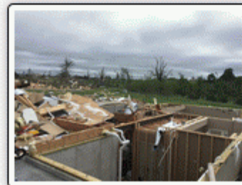
EF-3 damage to a home near Linwood, KS (NWS Survey).
